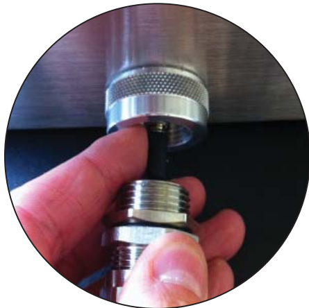
BOS SAFETAP - Typical Install at 4401OXY Analyzer
